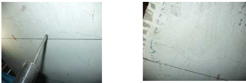
Figure 3.54 Cracks at the mid-span and along the line of application of load
